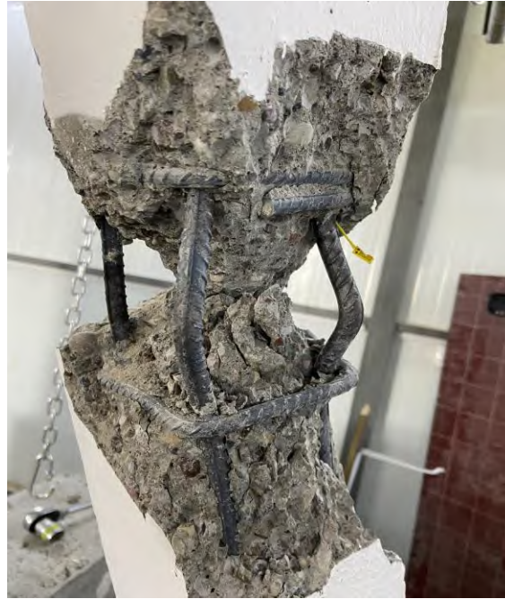
Figure 4.2: S-RA50Vf0E0 after failure
