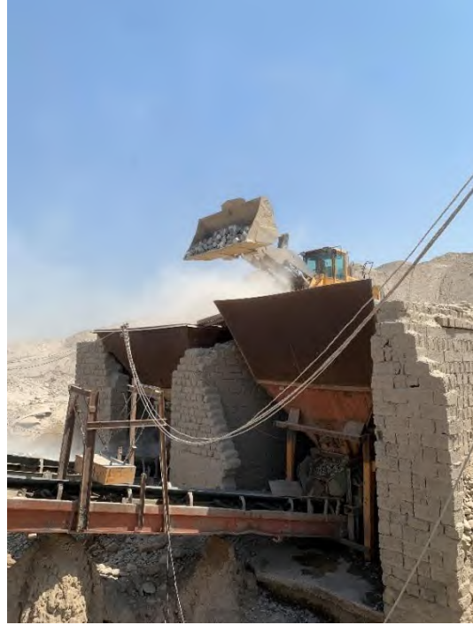
(b) Crushing of concrete
