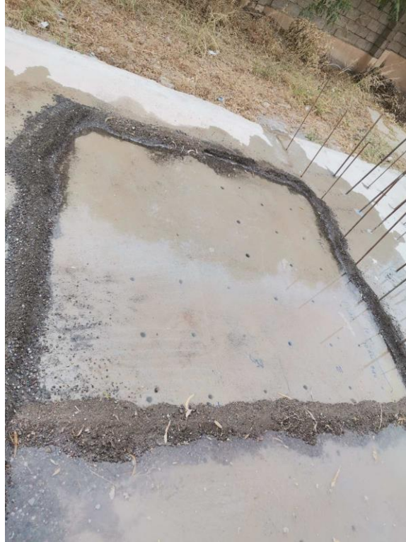
Fig. 3- 14 Drilled holes filled with water to provide saturated surface for the grouted anchors
