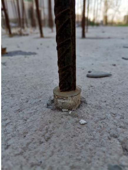
A) Concrete -adhesive interface (Mode 3)
