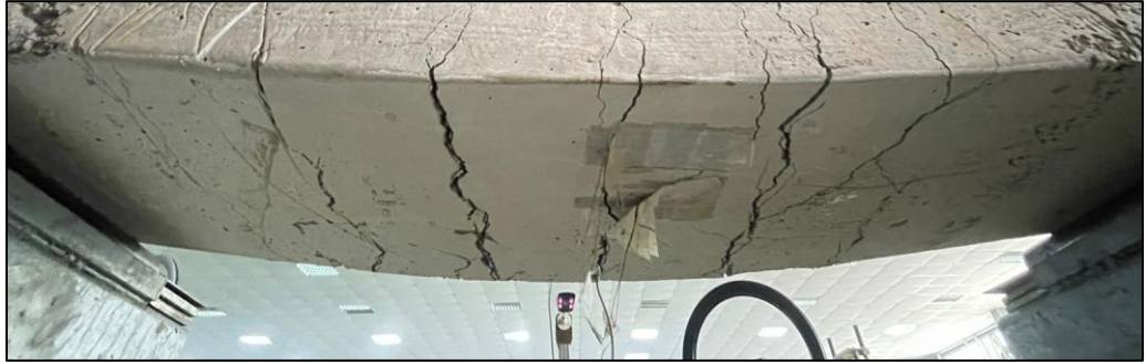
Figure 4.31: S21 mold Crack pattern
