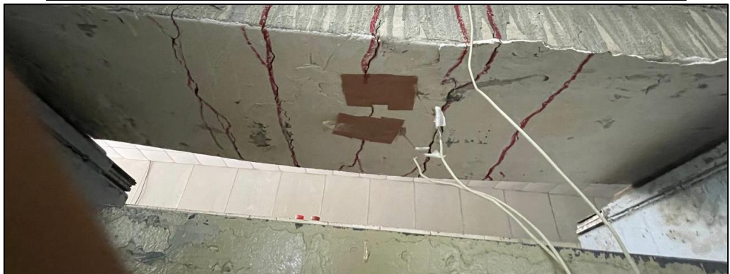
Figure 4.34: O80 mold Crack pattern
