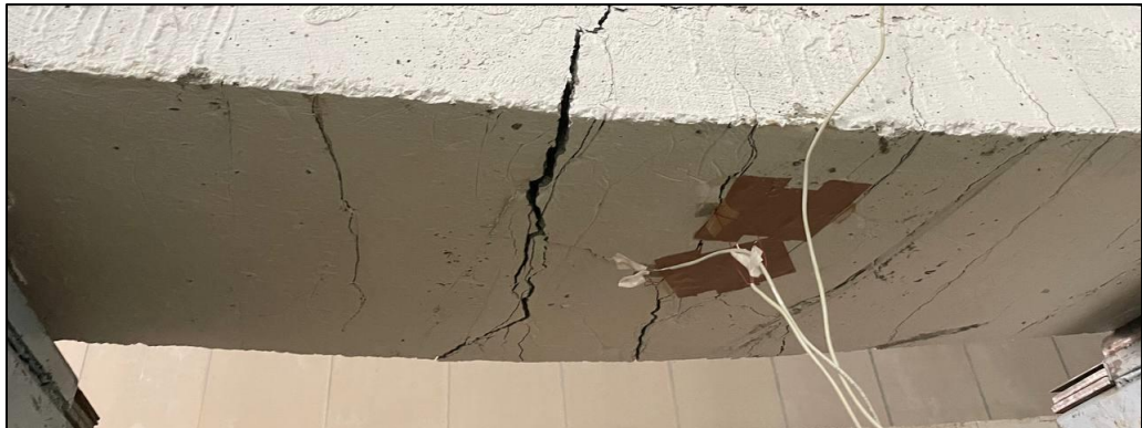
Figure 4.24: R-UHPC5 mold Crack pattern
