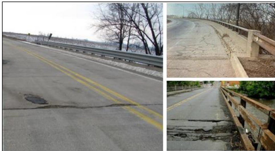
Figure 1.2: Examples of bridge deck slabs deterioration
