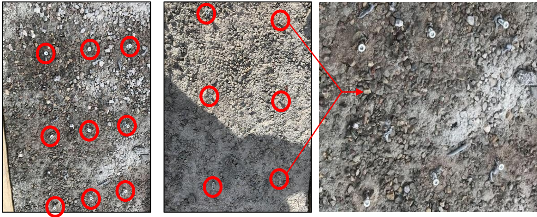
Figure 3.8: Anchor bolt embedded into the substrate concrete, (Left: three rows at 228 mm) and (Right: two rows at 228 mm)
