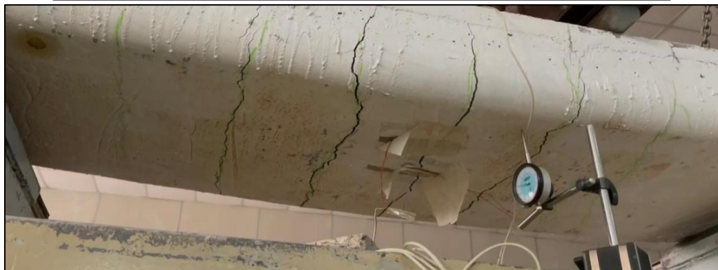
Figure 4.22: TH40 mold Crack pattern
