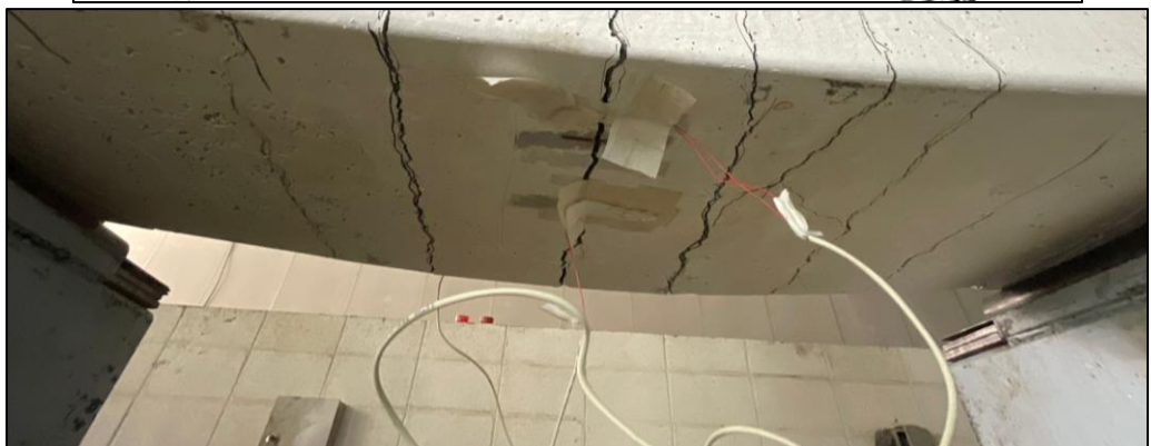
Figure 4.32: S40 mold Crack pattern
