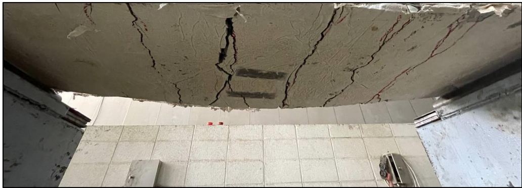
Figure 4.23: TH50 mold Crack pattern
