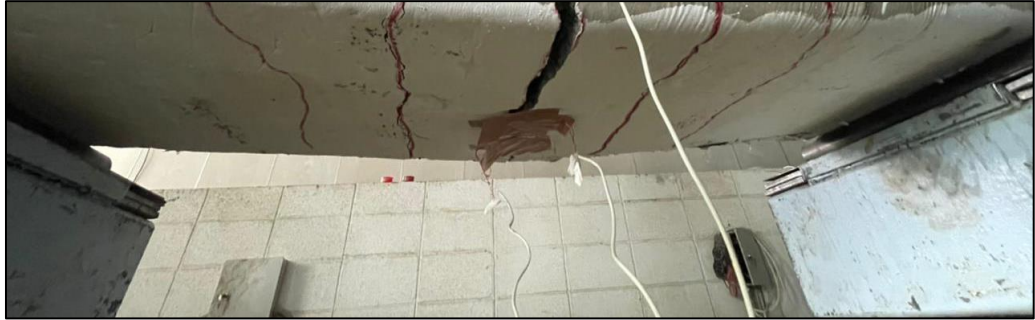
Figure 4.33: O30 mold Crack pattern
