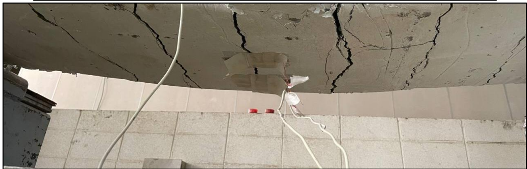
Figure 4.29: CH mold Crack pattern
